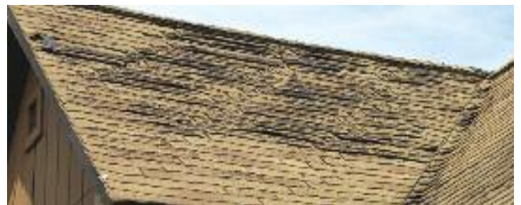
Our roof in much need of replacement!
